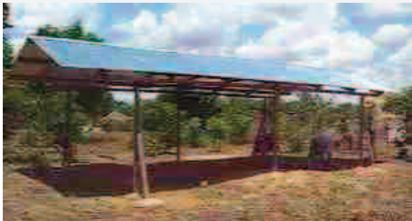
Photo: Roof for new two room school provides shelter for villagers to make bricks during the rainy season.
