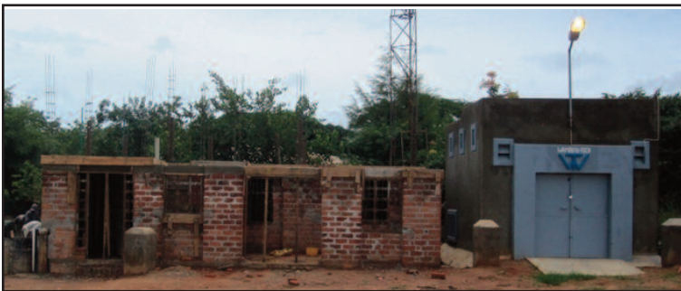
An office building (left) is being built next to the substation (right) on Myrt 1 campus. The office will be the regional headquarters for the power company and will insure that new hookup charges will be properly accredited to investors in the electrification project.
