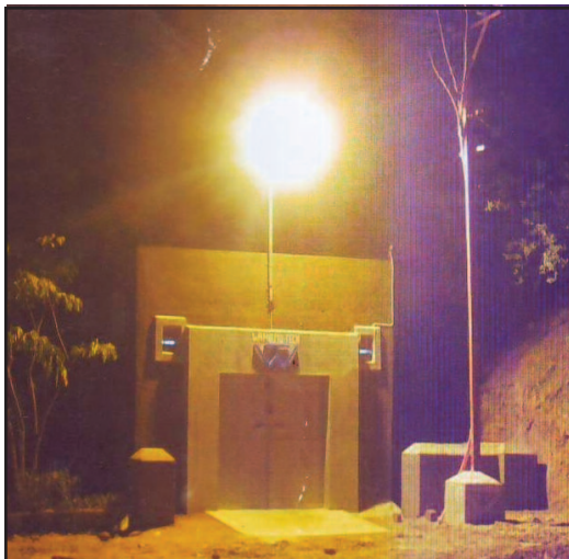
This electric substation on Myrt 1 Campus supplies economical green power to the campus and lights up the night.
